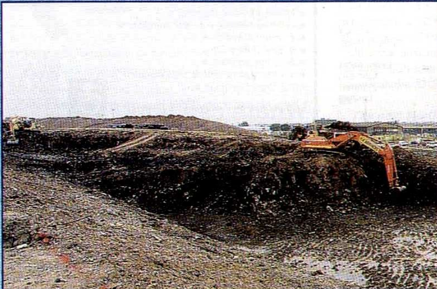
These pictures from Bob Lowery of Cloud 9 Photography show how work at the new stadium site is progressing.
